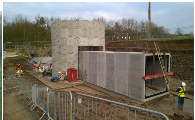
Control Structure on the South Site
