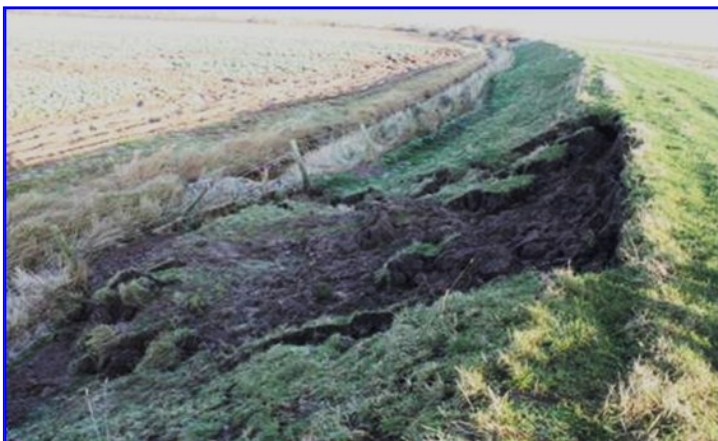
Photo of 2013 overtopping damage to sea banks
